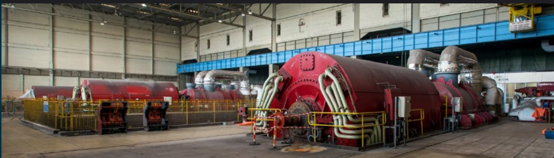
Uskmouth Power Turbine Hall showing 121 MW Turbines
