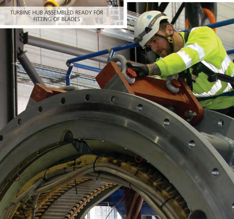
TURBINE ASSEMBLY AND TESTING IS UNDERWAY AT THE OFFSHORE RENEWABLE ENERGY CENTRE IN NORTHUMBRLAND
