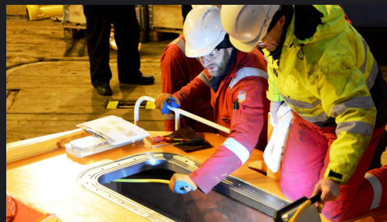
Lower cable management system connection
