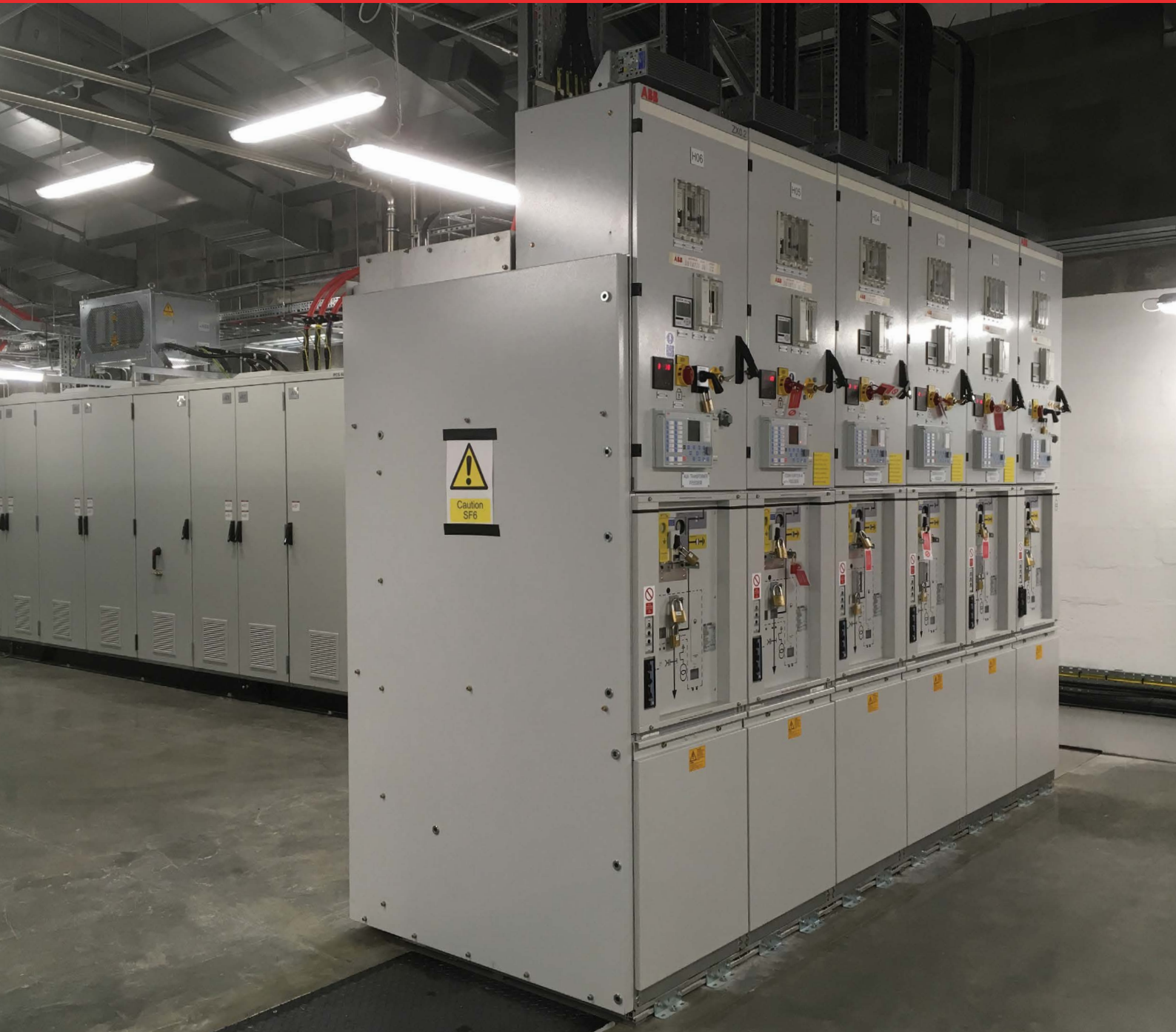
INSIDE MEYGEN'S POWER CONVERSION CENTRE AT NESS OF QUOYS, CAITHNESS
